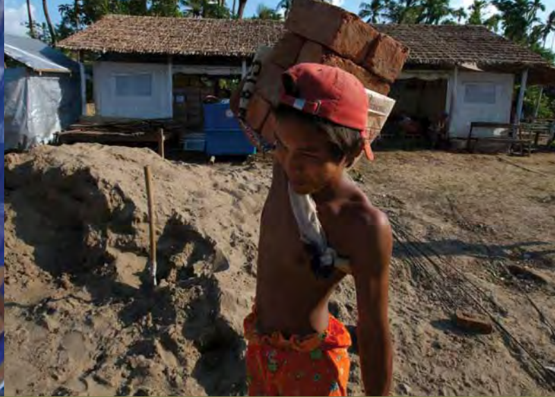
▲ Builders start work on a permanent rural health centre next to the KCCP tent clinic. © IOM 2008 - MMM0346 (Photo: Piers Benatar)
